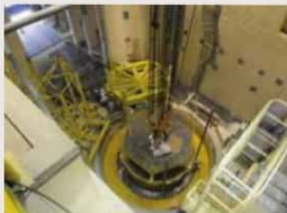
Interior de la Central Nuclear Atucha II.
